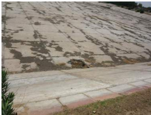
Figure 17.4 Hole in lining of facultative anaerobic pond.
